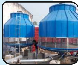
Cooling tower & Boiler Feed
